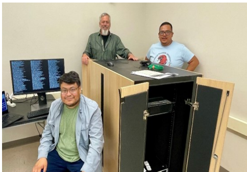
Figure E. Computer server installation for the SIPI Sovereign Data Network project. The project supports TCUs and tribal nations in realizing effective data sovereignty and governance.
